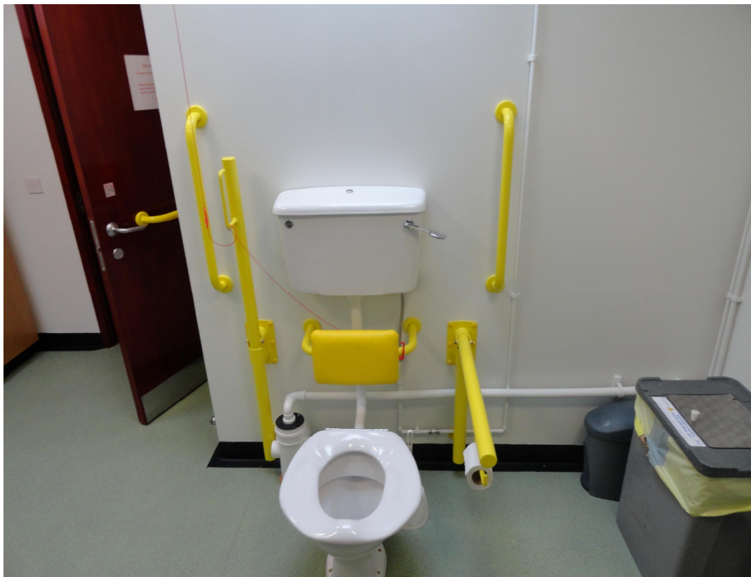
WC and colour contrasting grab rails
