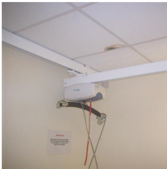
The fixed ceiling tracking hoist
