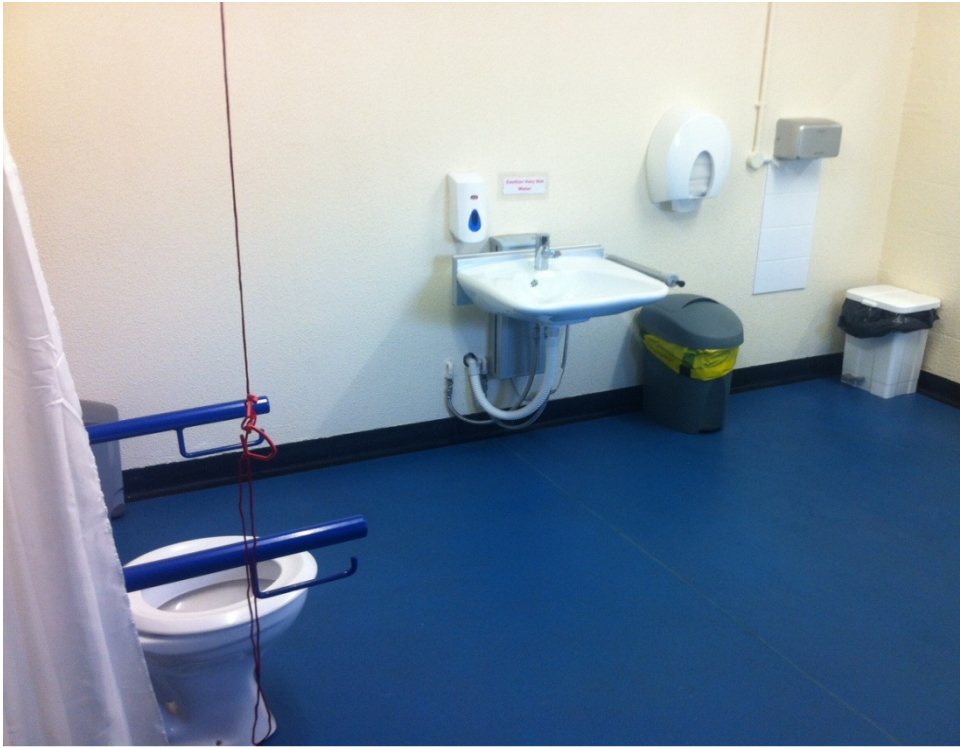
Spacious room and height adjustable wash hand basin
