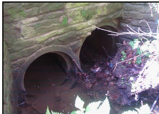
A partially obstructed culvert
