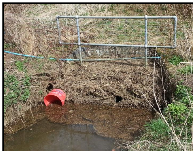
A blocked culvert
