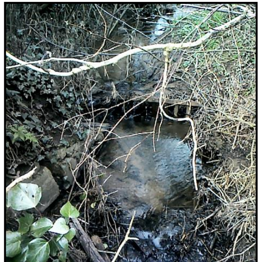
A partially obstructed trash screen
