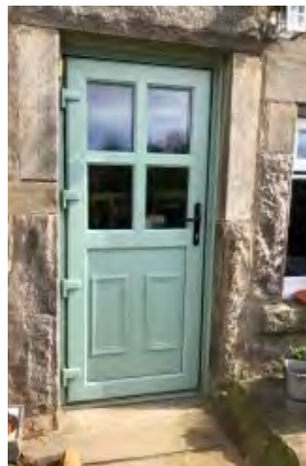
Flood door fitted.
