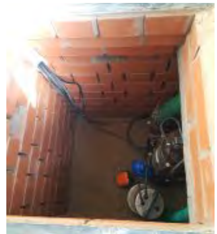
Two sump-pumps in lounge.
